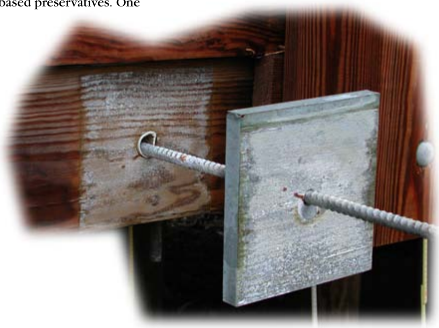
Figure 10—This metal plate used in a stress-laminated bridge constructed with preservative-treated wood shows the early signs of corrosion.— Photo courtesy of James Wacker
